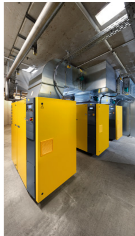
The compressed air station played a large part in the successful plan.
