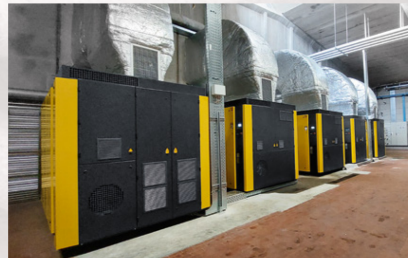
Image left: Cervotessile is renowned for its high-quality products that are rich in traditional history. Image right: The new compressed air station comprises five rotary screw compressors from KAESER.
